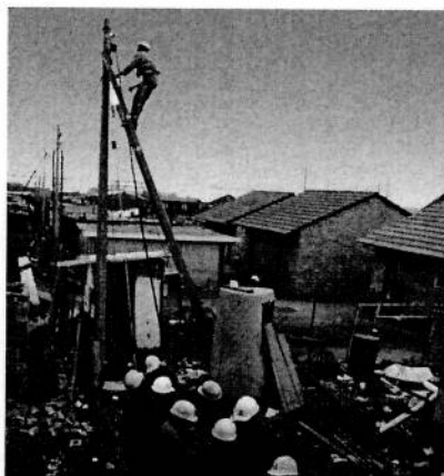
Eskom contractors stringing a power line which will supply electricity to the residential area in Orange Farm.
