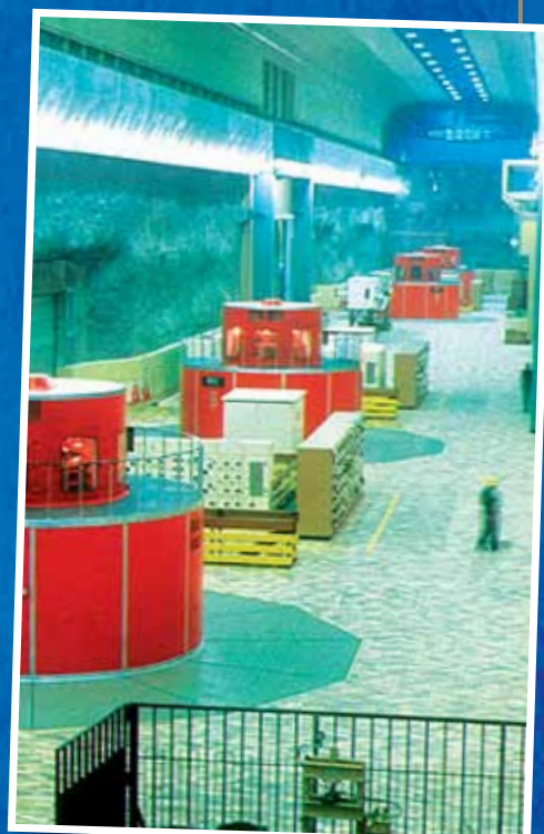
The machine hall at Drakensburg Power Station.
