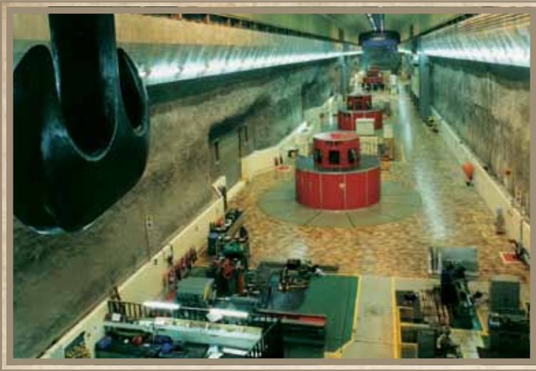
Drakensberg Pump Station
