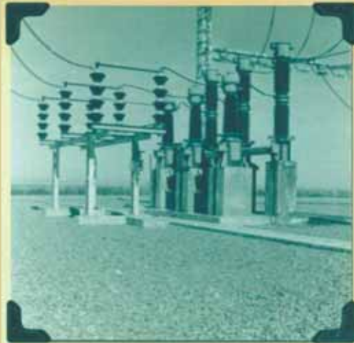
132kV feeder bay
