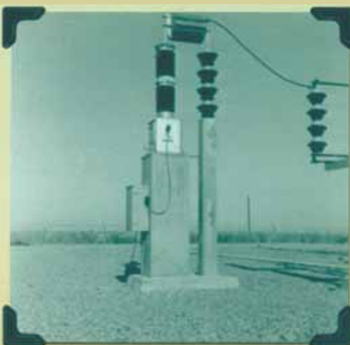
132kV Line trap and coupling capacitor
