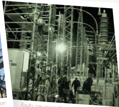
Faults can occur at any time during the day or night. Here, employees are repairing a breaker at 4 o'clock in the morning at Bacchus Substation.
