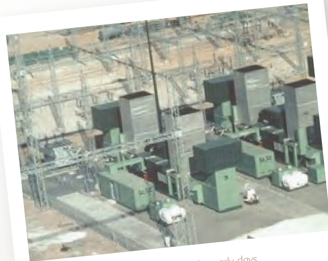
Acacia Power Station, the early days
