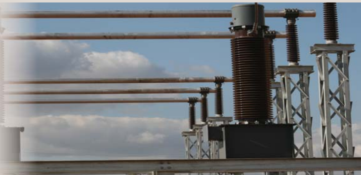
Top: Construction of Medupi power station is advancing well. Bottom: Insulators in the new 132kV yard at Medupi.
