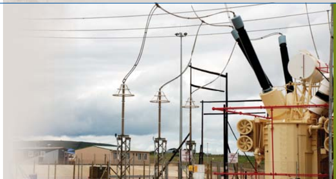
A typical transformer at a substation next to a power station.
