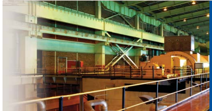
The turbine hall at Duvha power station near Witbank.
