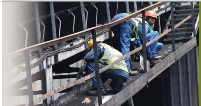
Workers remove wet coal jamming conveyor belts at Duvha power station.
