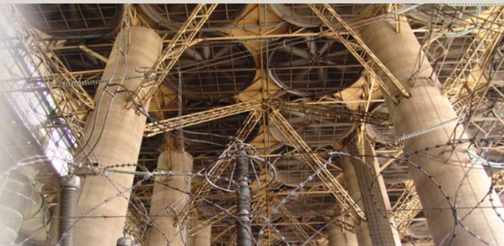
The cooling fans at Matimba power station in Lephalale.
