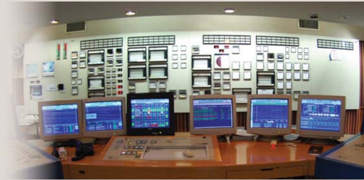
The control room at Kendal power station.
