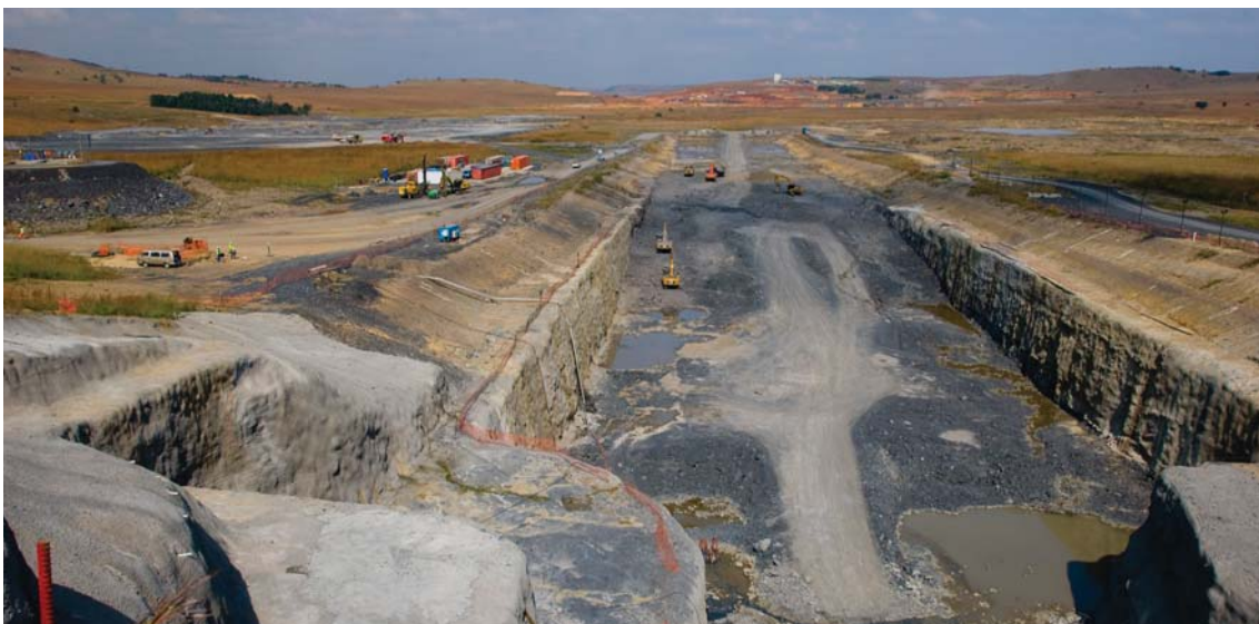
Construction of the two dams at Ingula pumped-storage scheme is progressing well
