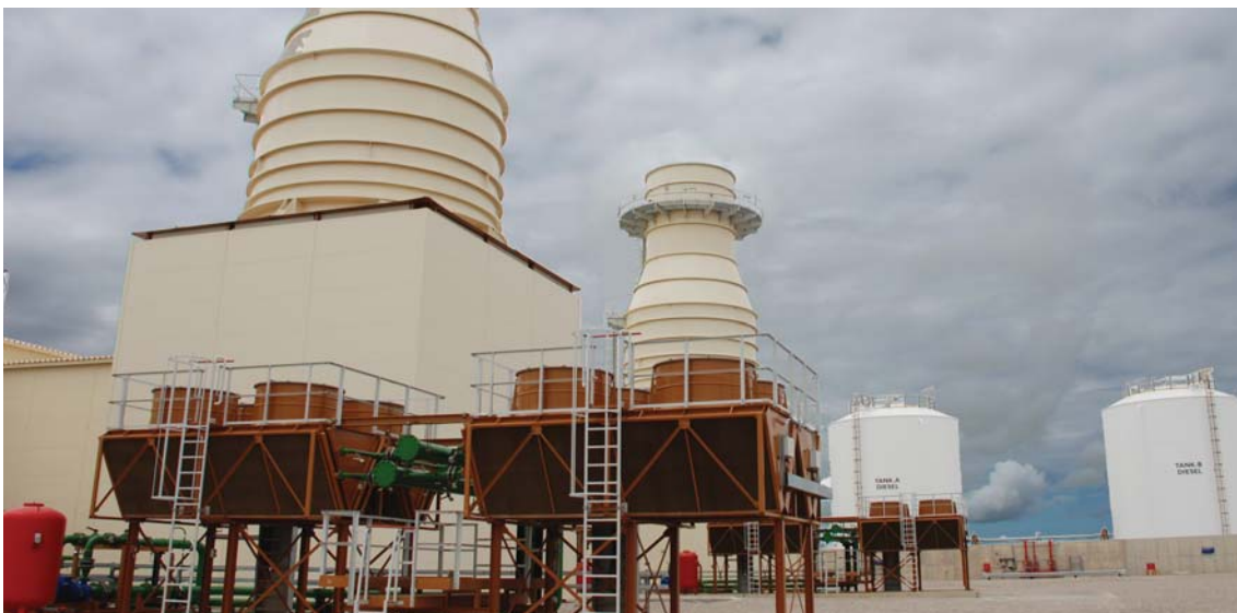
The Gourikwa open cycle gas turbine station was used less often to reduce fuel costs
