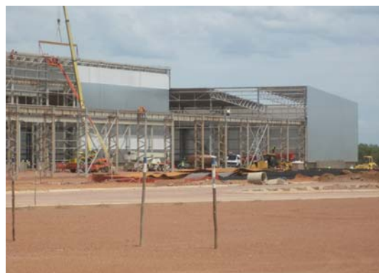
Unit 6 of the new Medupi power station in Lephalale
