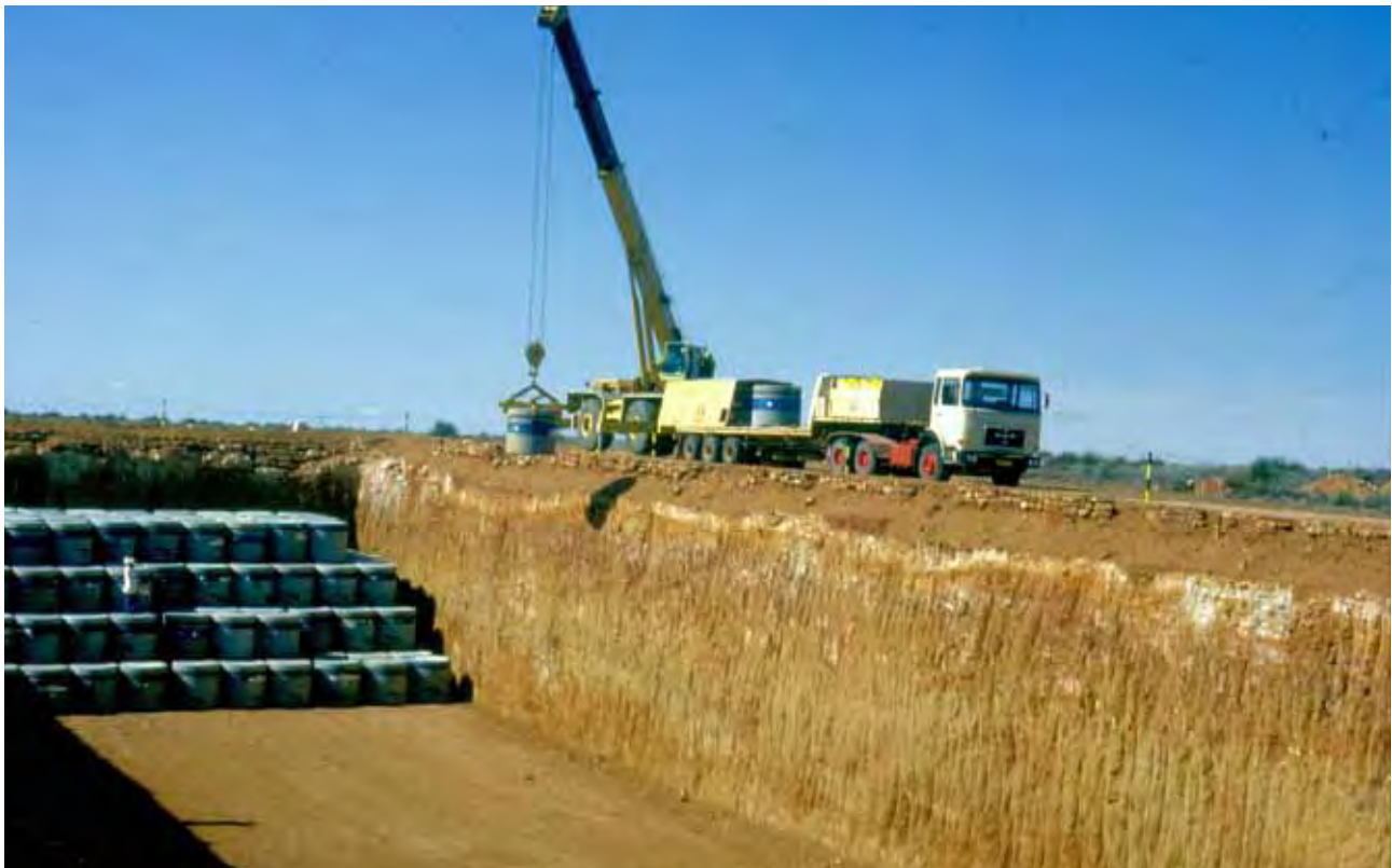
Low-level waste is stored in steel drums at Vaalputs waste disposal site in the Northern Cape.
