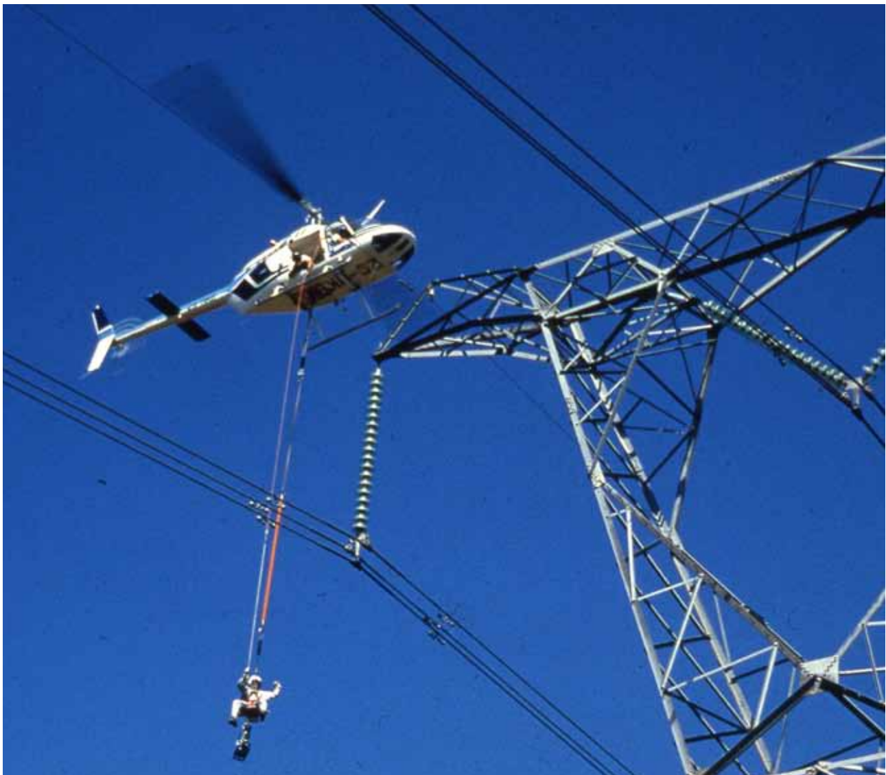
Liveline teams maintain high-voltage lines under live conditions to reduce inconvenience to customers.
