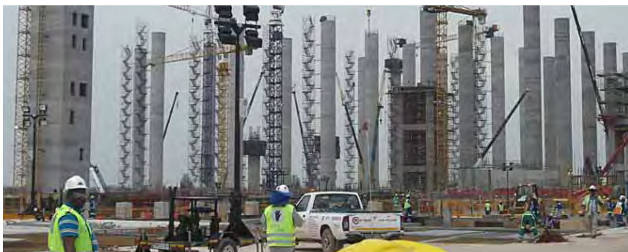
Construction of the Medupi power station in Lephalale, Limpopo province, is well advanced.
