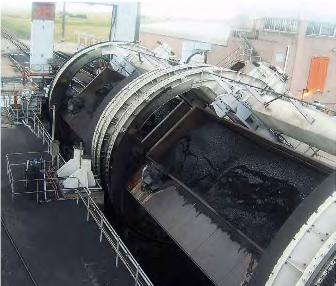
Train downloads coal at Majuba power station near Volksrust.
