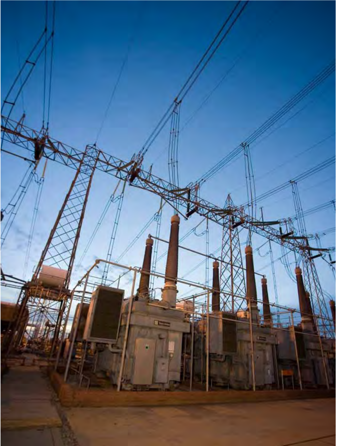
Apollo substation in Gauteng is the main interconnection to Cahora Bassa in Mozambique.
