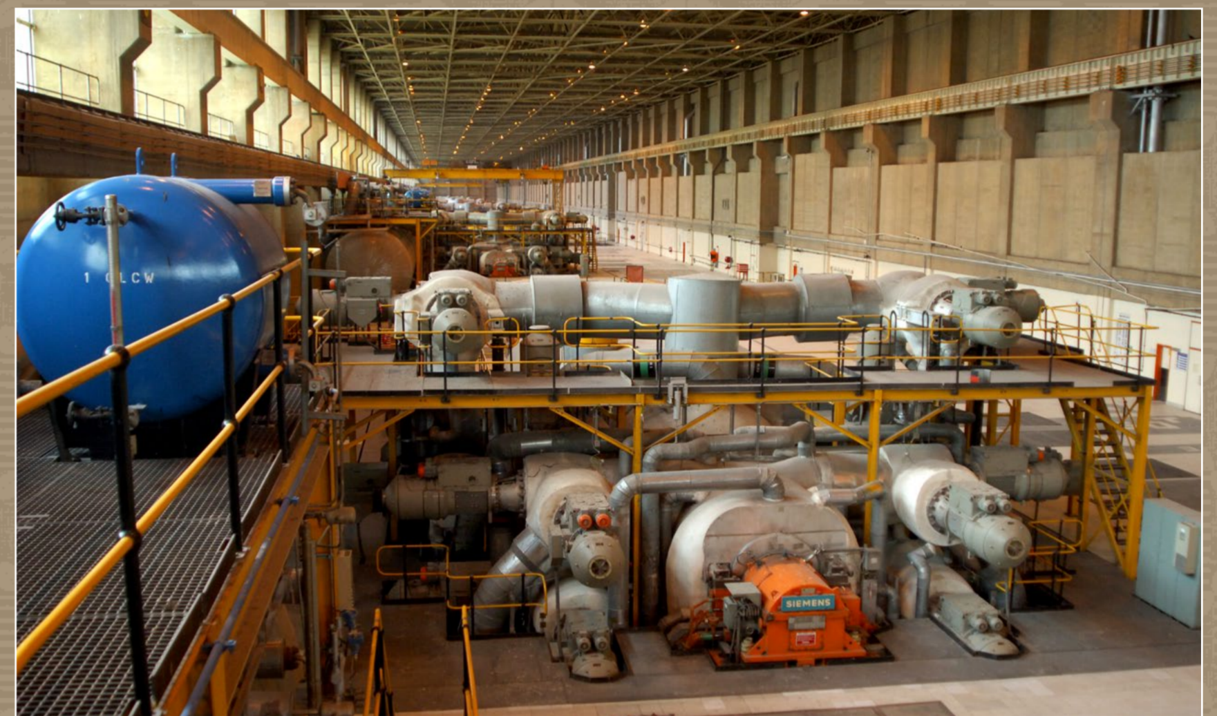
Duvha Power Station
