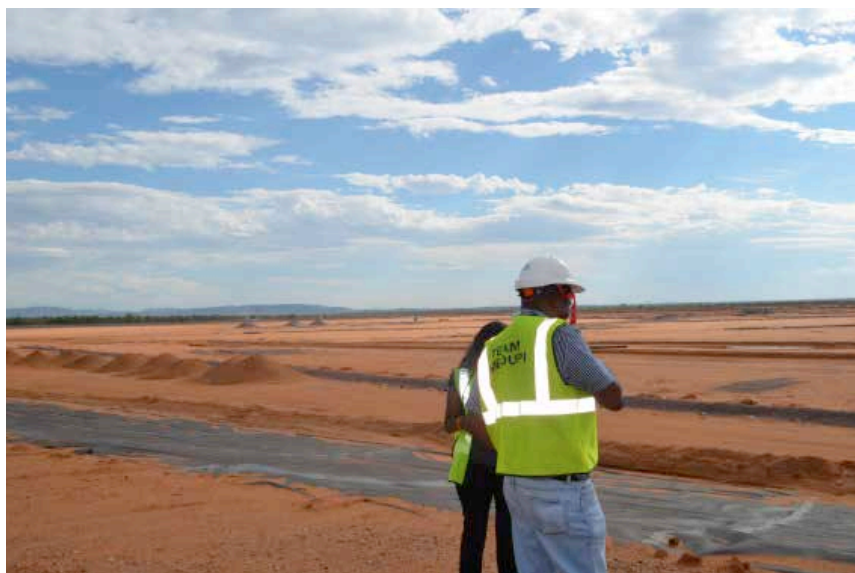
The newly constructed ash dam at Medupi power station is funded by the World Bank
