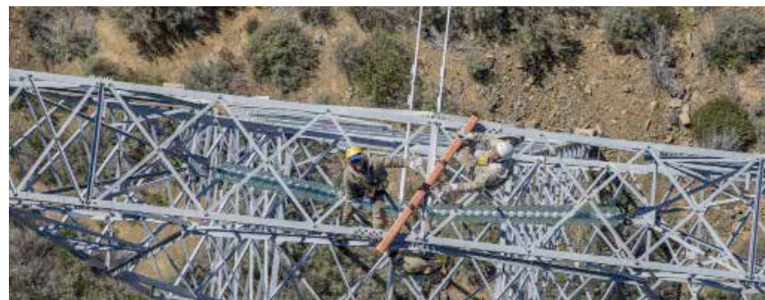
Live-line maintenance on the high-voltage powerlines ensures a healthy national power grid
