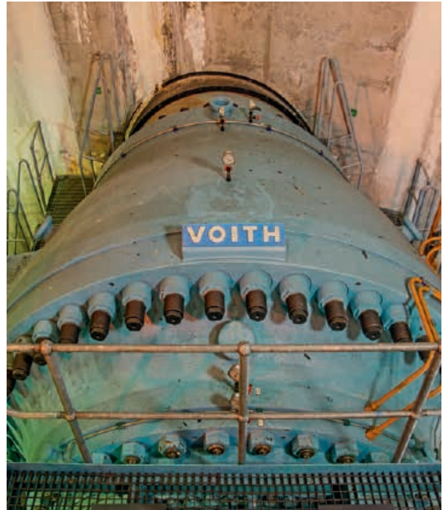
Routine maintenance at the Palmiet pumped-storage scheme near Grabouw in the Western Cape
