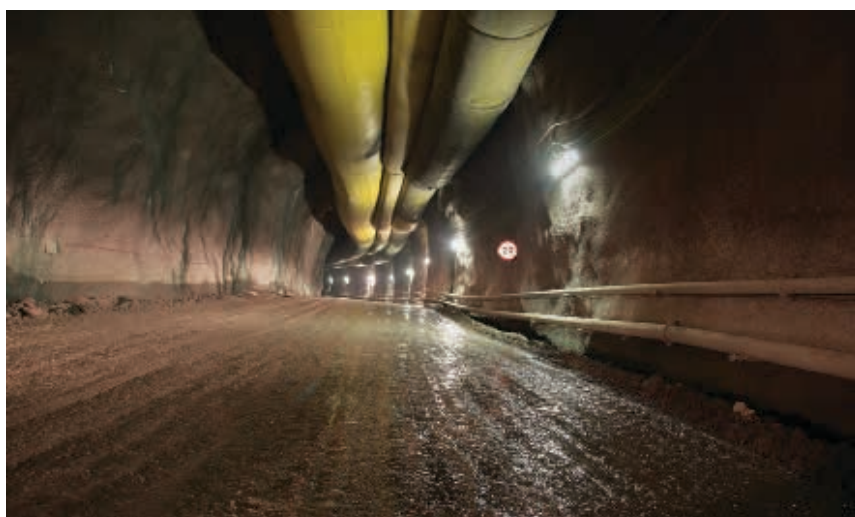
The Ingula pumped storage scheme under construction entails 16km of tunnels and 8km of waterways
