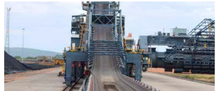
The new coal conveyor at Medupi power station measures 5.2km in length to the Exxaro mine
