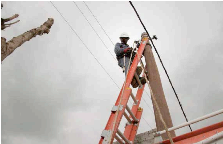
Regular maintenance strengthens the distribution network
