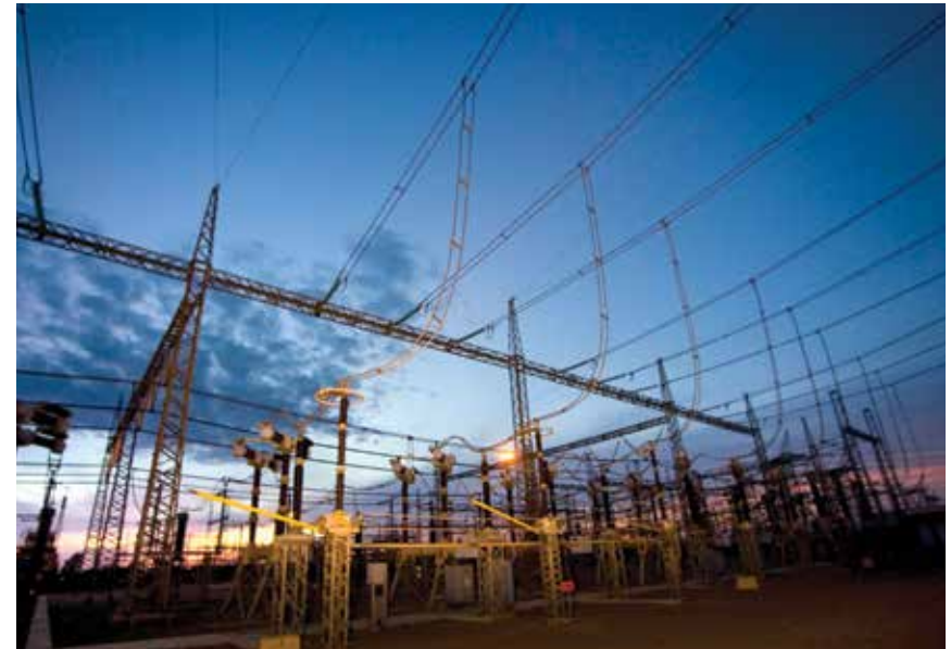
Eskom has commissioned a total of 27 565MVA substation capacity since 2005
