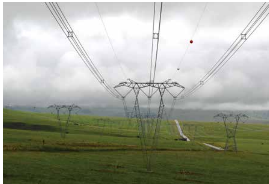
The 94km high-voltage line from the Ingula pumped-storage scheme to the Venus substation has been completed
