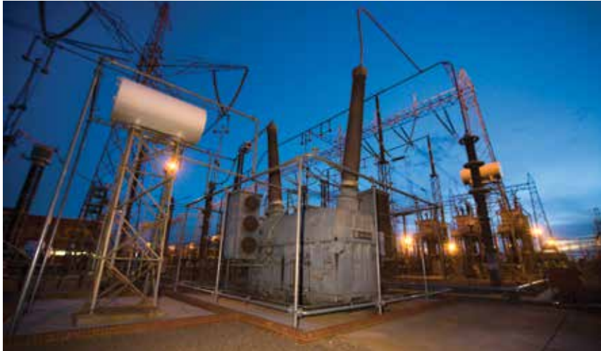
The Apollo HVDC converter station in Johannesburg converts the direct current power into alternating current power from Mozambique and then feeds it into the South African national grid
