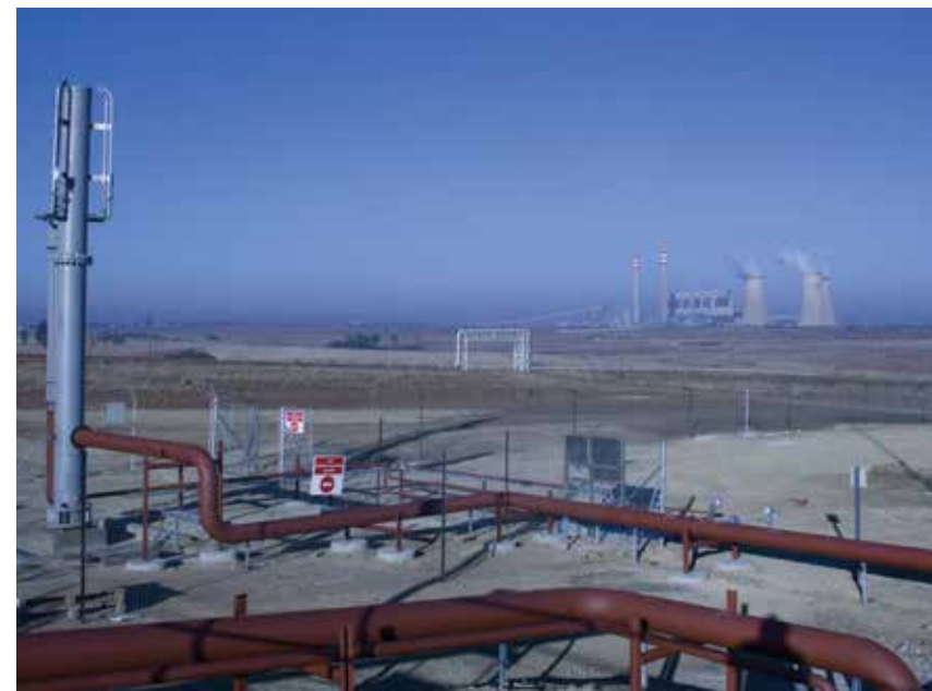
The underground coal gasification project next to the Majuba power station has been a highlight in Eskom's research portfolio
