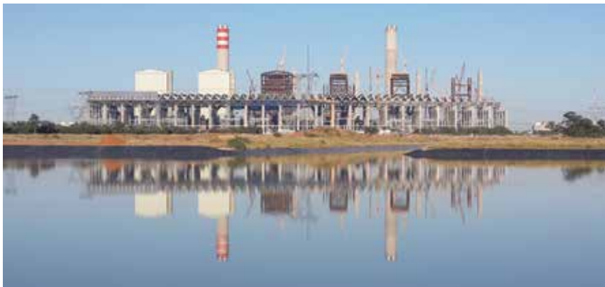
Construction at the Medupi power station as seen from the clean water dam
