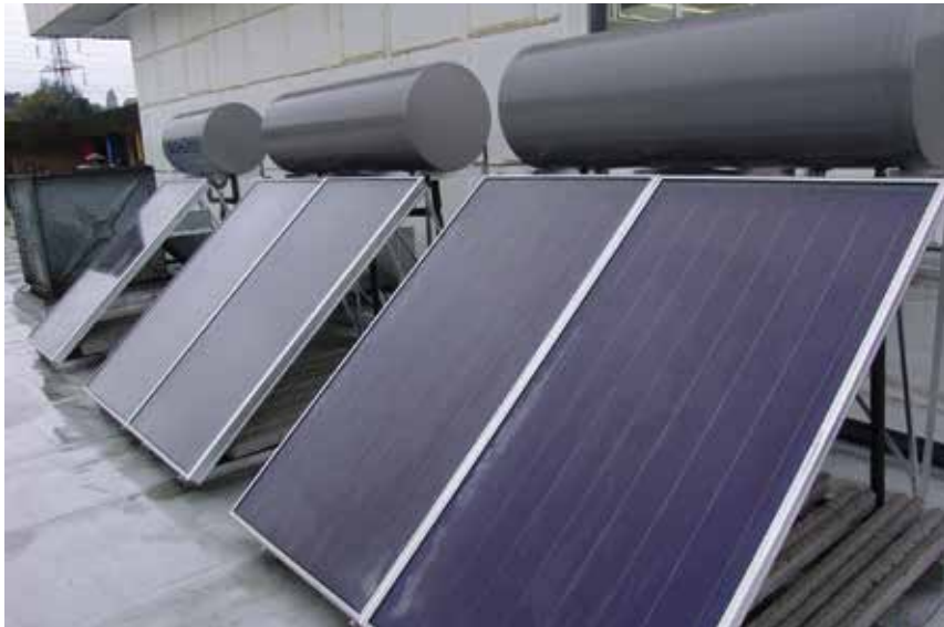
Eskom contributes to the government's solar water heating initiative, which aims to install one million solar water heaters
