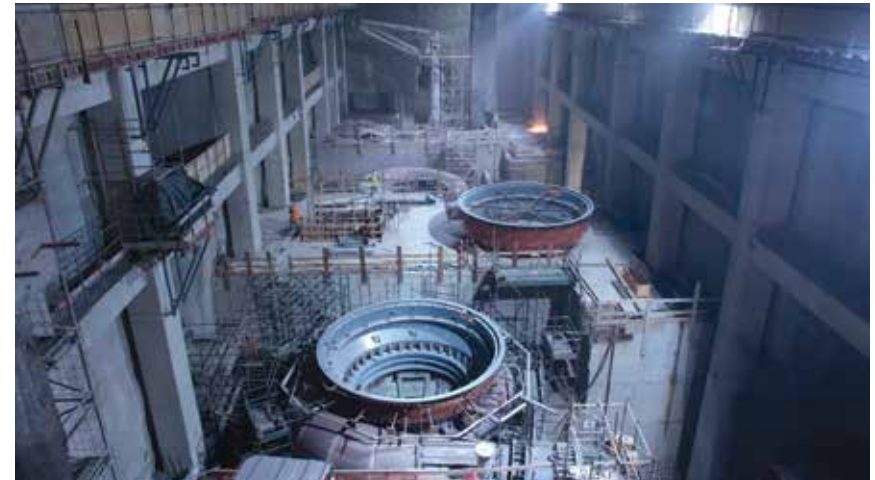
The machine hall at the Ingula pumped-storage scheme project is the largest cavern in mud rock in the world
