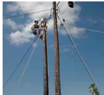
The maintenance of over 48 000km of distribution power lines across South Africa requires strict adherence to safety regulations
