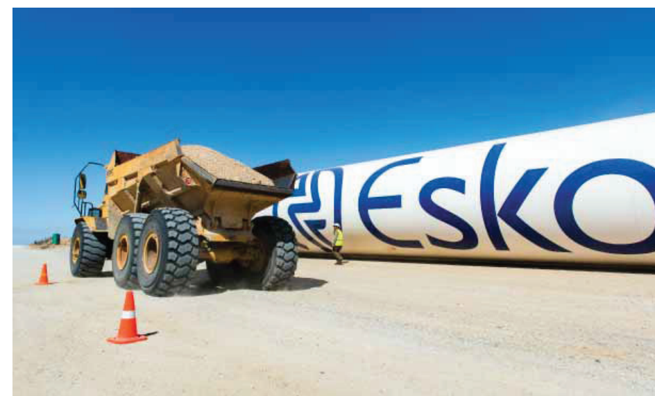
One of the turbine masts at the 100MW Sere Wind Farm, our first utility-scale renewable energy project, which was placed into commercial operation on 31 March 2015
