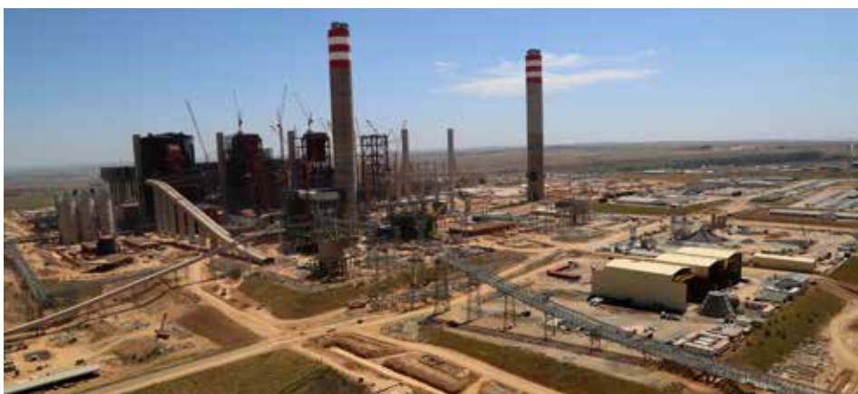
The Kusile project continues to achieve set milestones, on track for commercial operation of Unit 1 by the second half of 2018. Good progress is also being made on Units 2 to 6.
