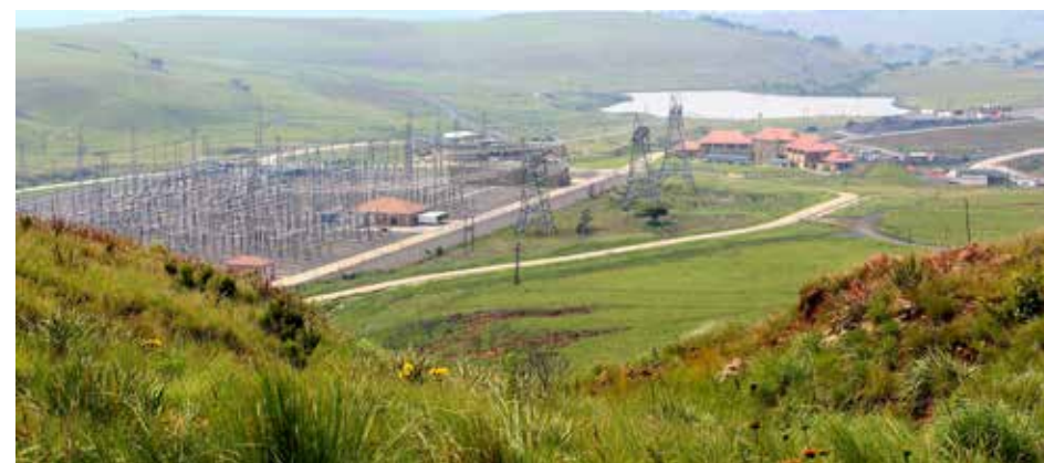
Units 3 and 4 of Ingula Pumped Storage Scheme were synchronised to the national grid in March 2016, with commercial operation of these units being planned for the 2016/17 financial year. (Photo: Heidi Pieterse)
