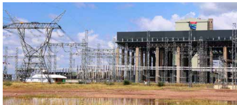
The HV yard at Medupi assists in evacuating energy sent out by Unit 6 to the national grid.
