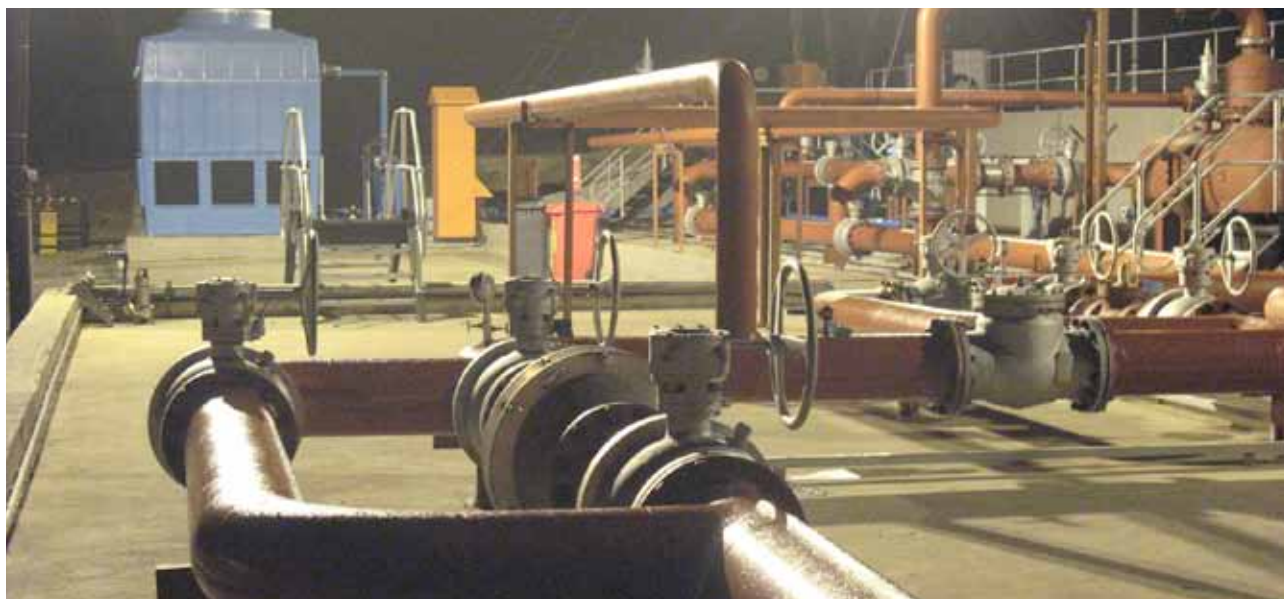
The piping of the underground coal gasification project next to the Majuba power station near Volksrust
