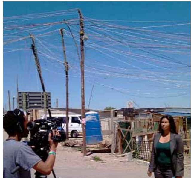
Illegal connections in residential area
