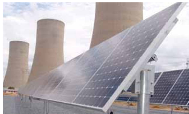
This year a photovoltaic installation was erected at Lethabo Power Station as part of Eskom's commitment to renewable energy
