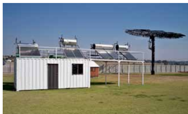
Solar heater test facility at Rosherville
