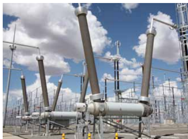
A high-voltage yard in the Free State
