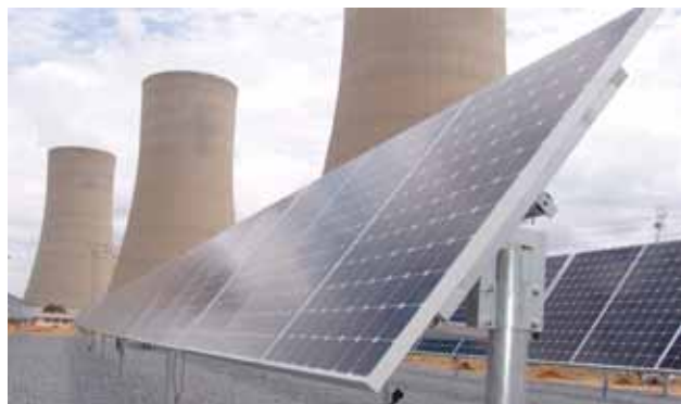
Photovoltaic installation erected at Lethabo Power Station
