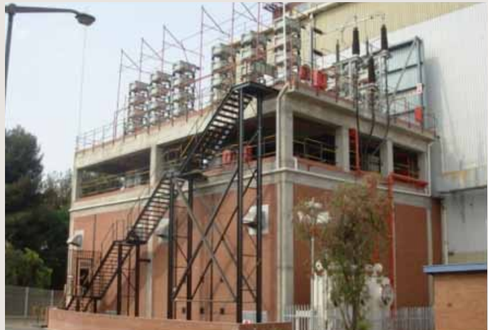
Rotek Industries, a subsidiary of Eskom specialising in the repair of transformers, opened its new transformer test bay facility in Rosherville, Germiston.
