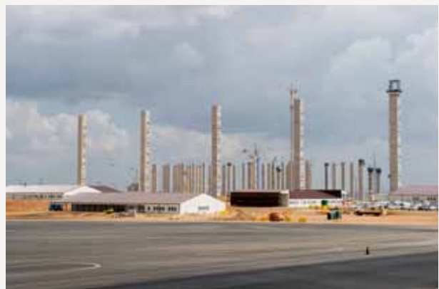
The new Kusile coal-fired power station with the site offices in the foreground.
