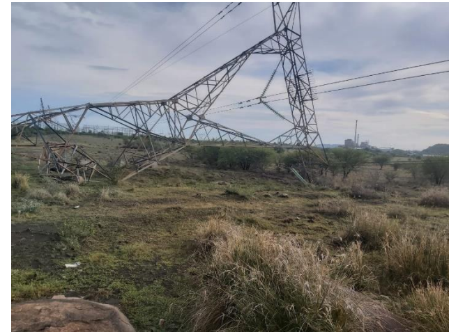
Pluto – Bighorn 400kV transmission line
