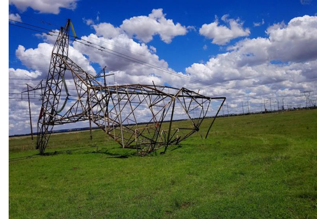
Hera – Westgate 275kV transmission line
