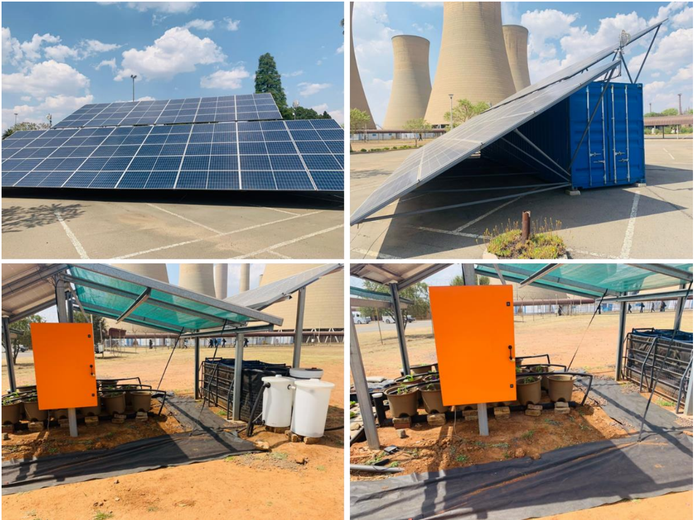
Picture 1: Demonstration Microgrids and agrivoltaics solutions at KPS
