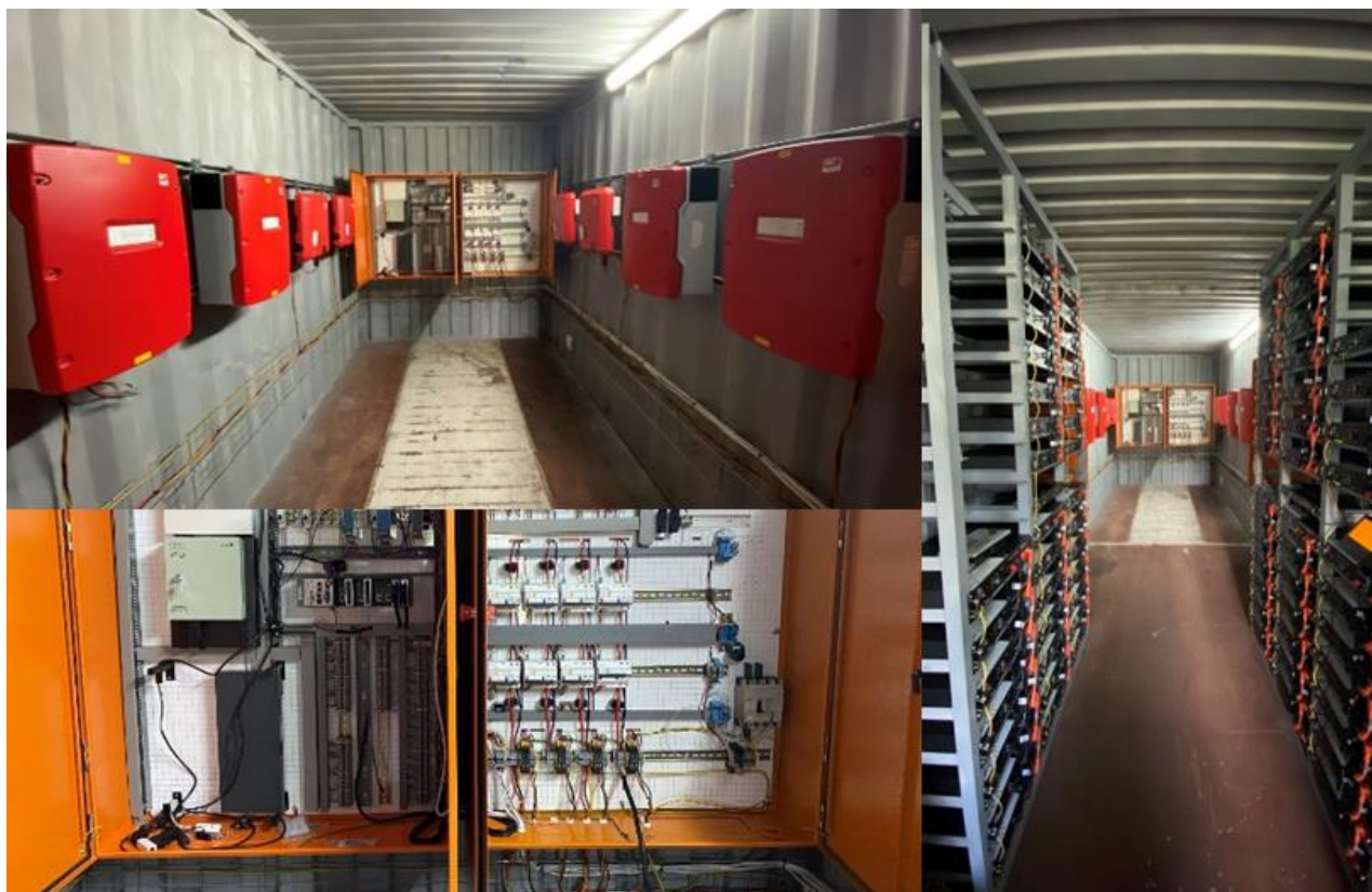
Picture 8.2: Control and communication systems and lithium-ion battery banks inside the container
