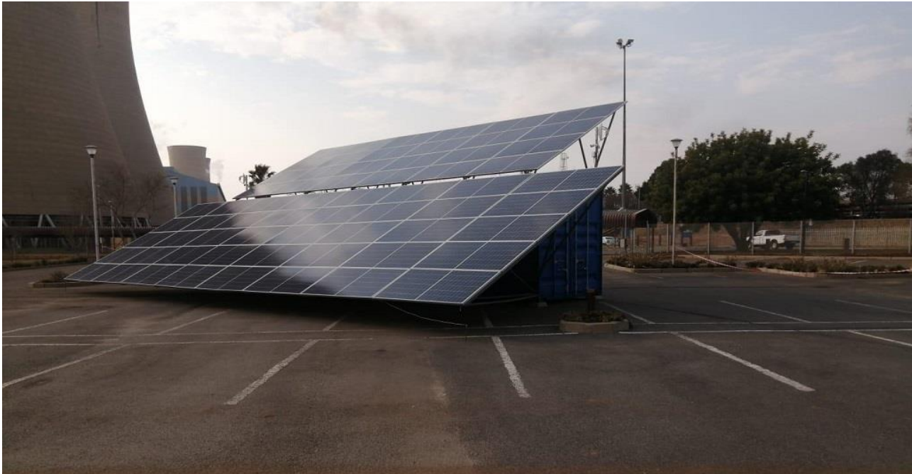
Picture 8.1: A containerised microgrid at KPS
