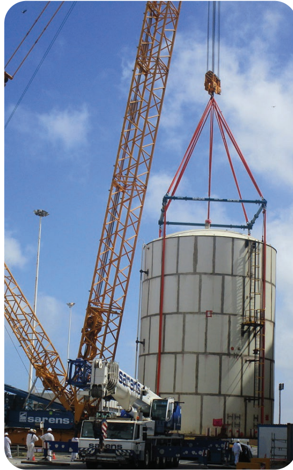
Reactor Cavity and Spent Fuel Pool Cooling System tank.
