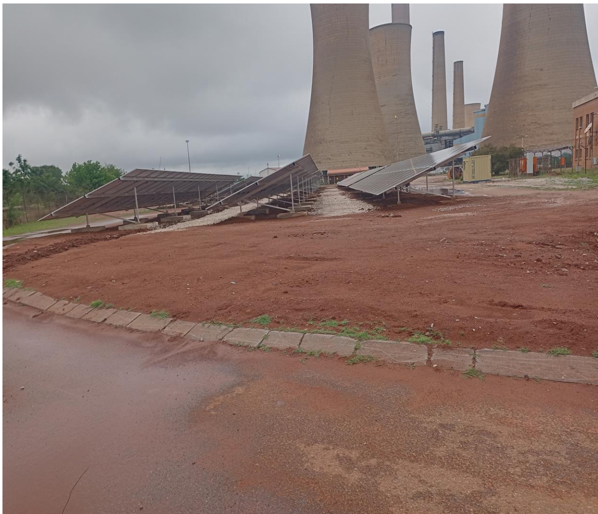
Photo 3: Agri-voltaic Plant at Komati Power Station
