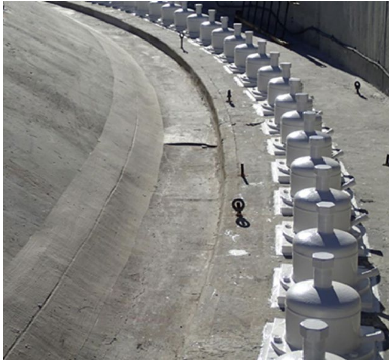
Figure 8: Containment dome crack sealed and coated
