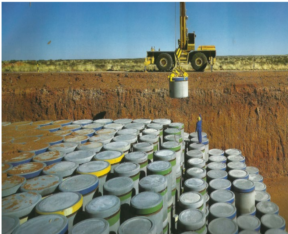
Figure 12: Radioactive waste in concrete waste drums stored at Vaalputs National Waste Disposal Facility
