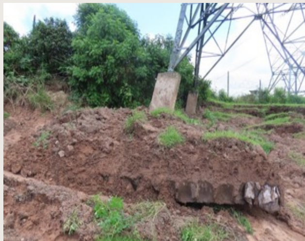
Mudslide and tower damage
