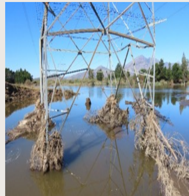
Foundation failure on the Durban South – Klaarwater 275kV Line
