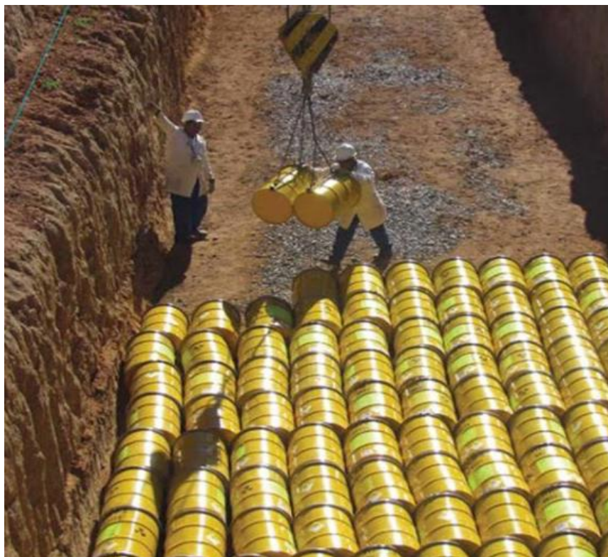
Figure 10: Radioactive waste in steel drums stored at Vaalputs National Waste Disposal Facility
