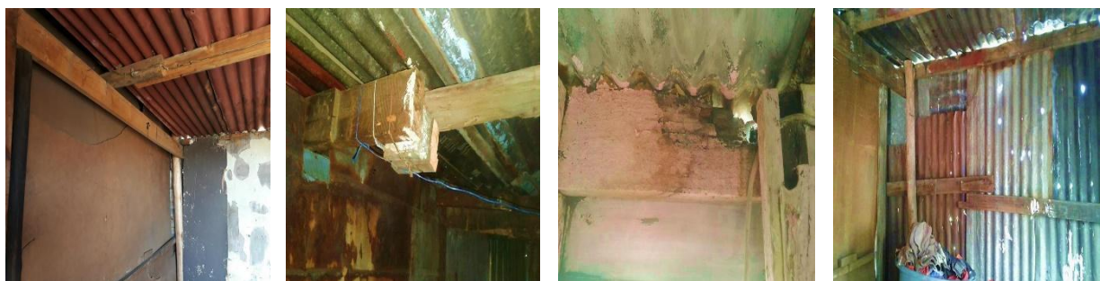
Figure 17 The wooden substructure of vertical poles and horizontal planks, clad with corrugated iron roof and Masonite inner walls (Nova Institute 2018).
