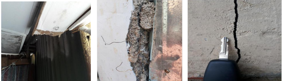
Figure 18 Post-insulation and ceiling damages
