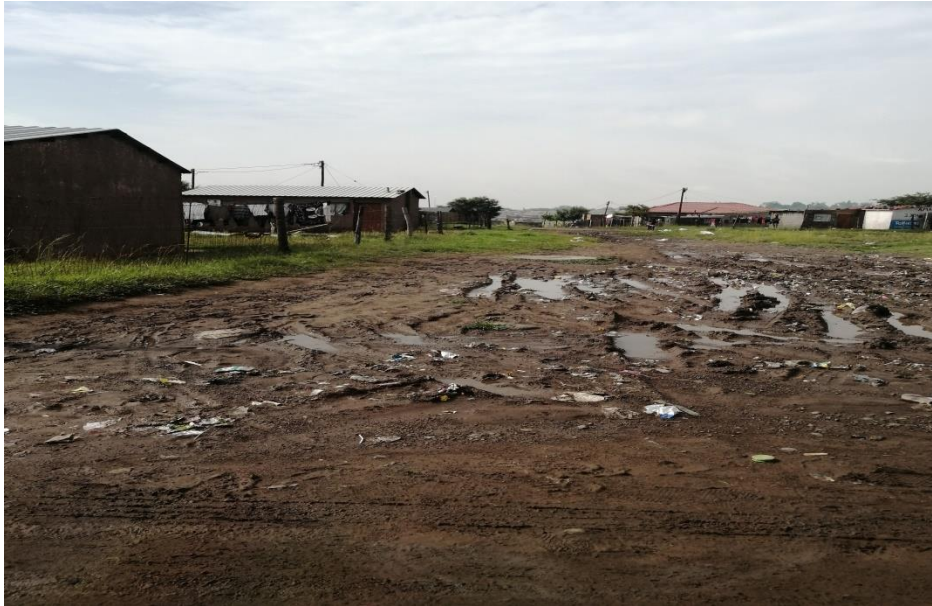
Figure 16: Road conditions in Ezamokuhle
