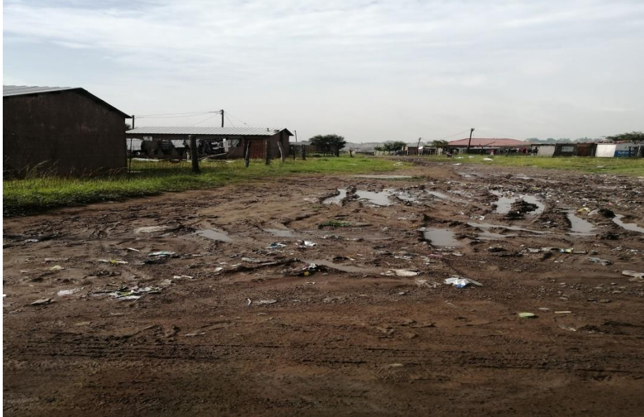
Figure 12: Road conditions in Ezamokuhle
