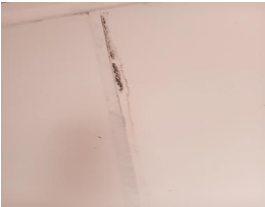
Image 1: Ceiling stains noted in household
