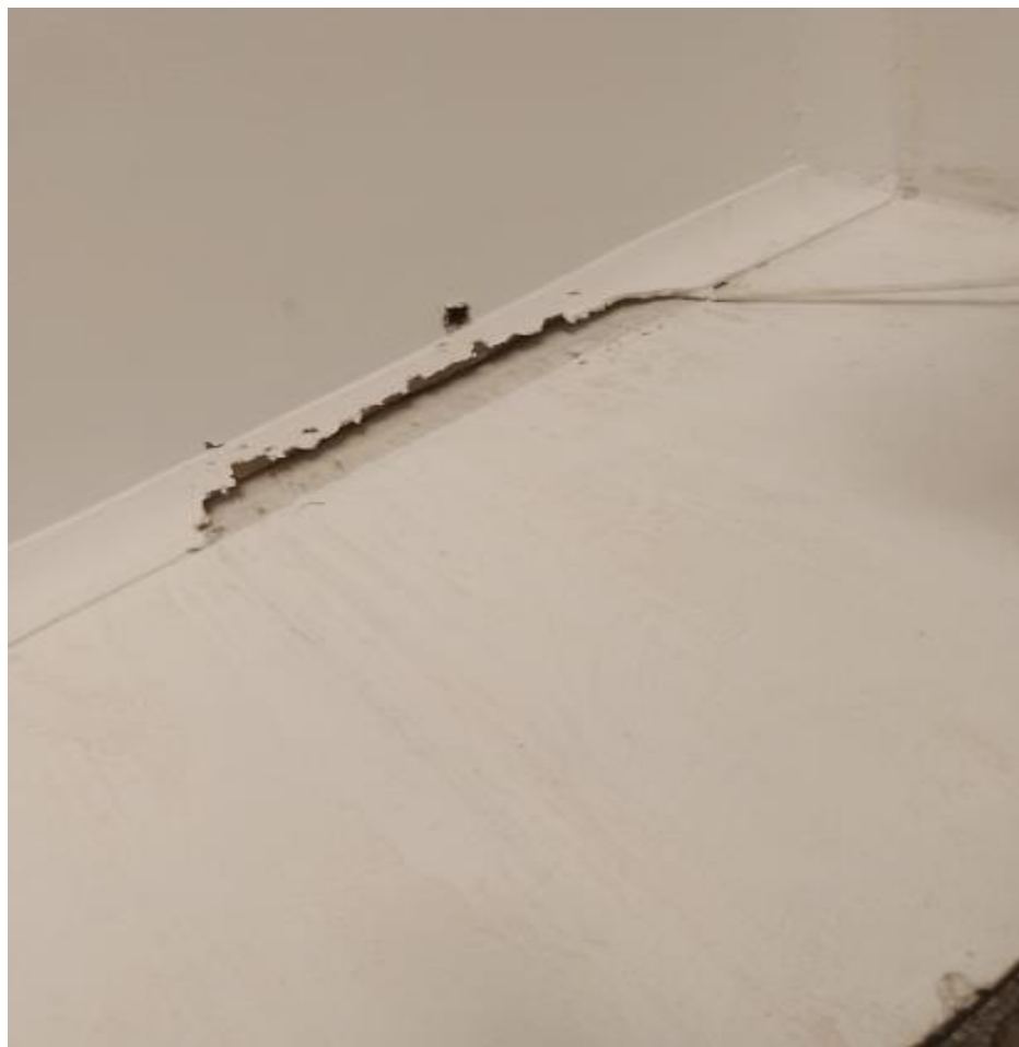
Figure 59: Loose cornice in a respondent's household
