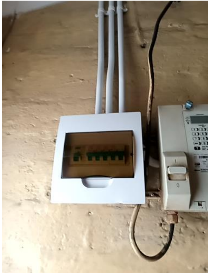
Figure 78:Example of wiring installed in households
