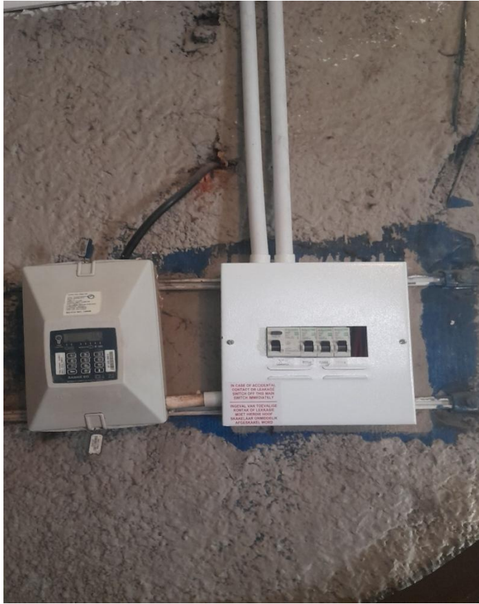
Figure 77: Example of wiring installed in households
