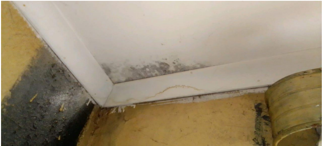
Image 1: Ceiling stains noted in household
