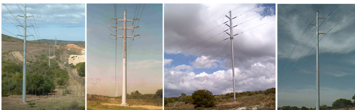
Figure 2.3: Examples of the proposed 132 kV monopole double circuit power line tower type.
