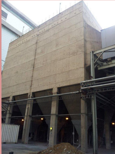
Figure 2: Existing Concrete ESP Casing within which the new Fabric Filter Plant will be installed, while extending the height of the casing with 1.1 meters.
