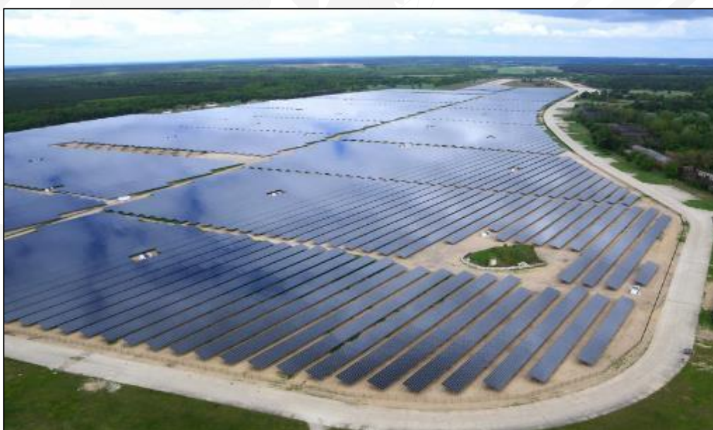
Figure 4: Solar PV Plant
