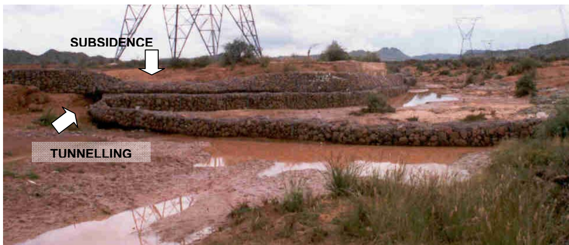
Figure 30: Subsidence of Gabion Structures following flooding [9]
