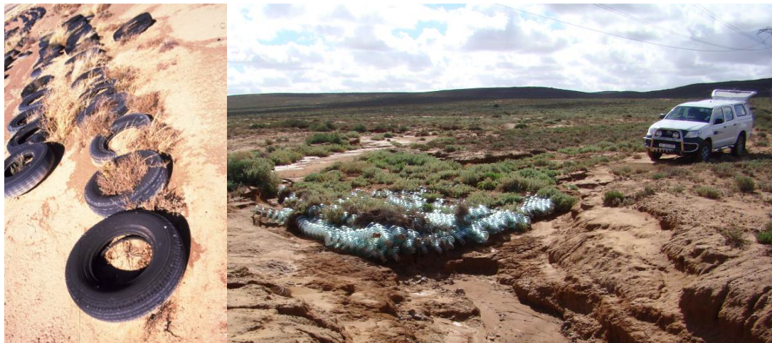
Figure 2: Use of waste material in erosion structures is not recommended [32]
