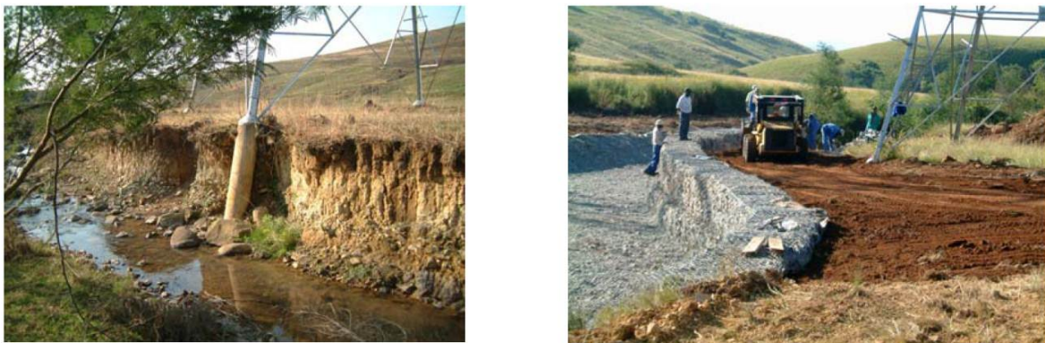
Figure 24: Before and after image of extensive gabion and reno mattress protection [5]
