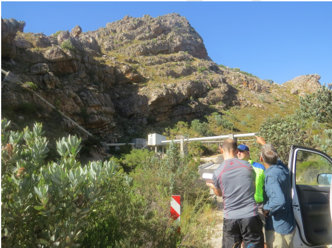
Figure 3-2: Above ground steel pipeline
