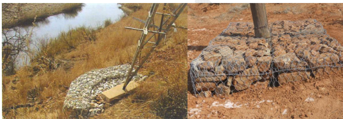
Figure 3-9: Gabion wall protecting tower leg and pole foundation (1)(2)
