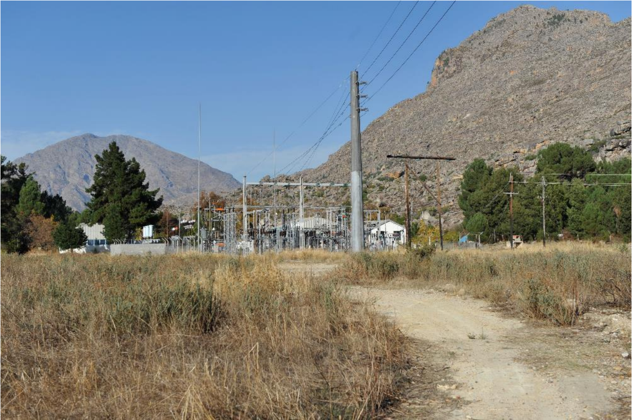
Figure 1: Industrial infrastructure (Ceres substation)
