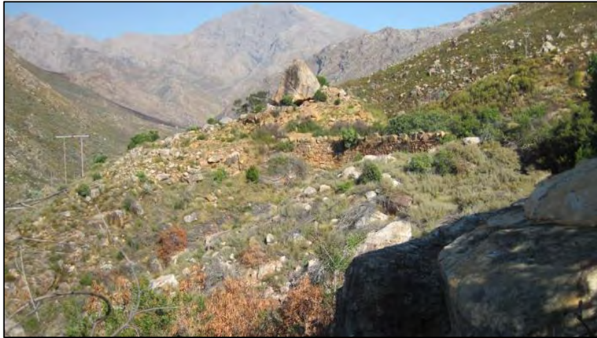
Plate 3.12: Looking back towards where Tower 057 will be erected. The embankment wall (D015) can be seen at right. The old 66kV powerline can be seen at left.
