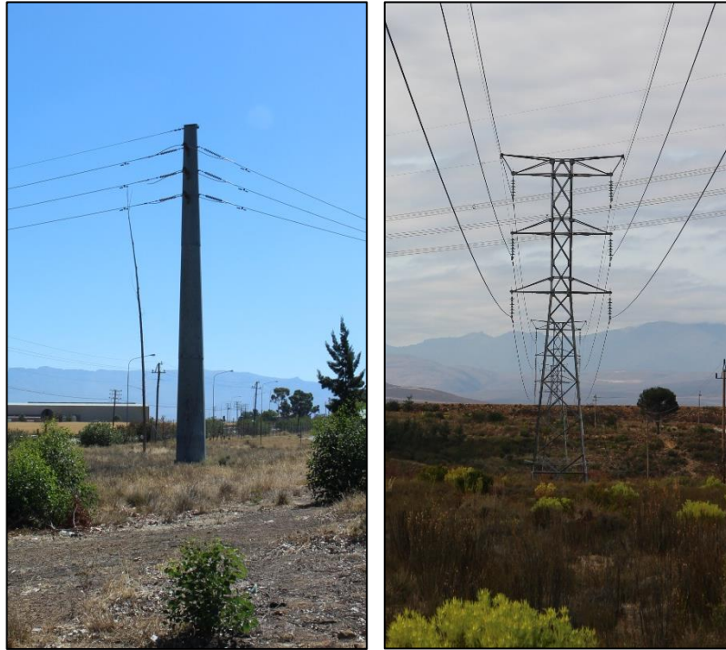
Figure 3-1: Indicative representation of the pylon types considered for the project - steel monopole (left) or steel lattice (right) pylons
