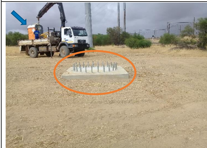
Figure 3: Completed and backfilled mono-pole structure. Arrow points to a chemical toilet being removed from site.
