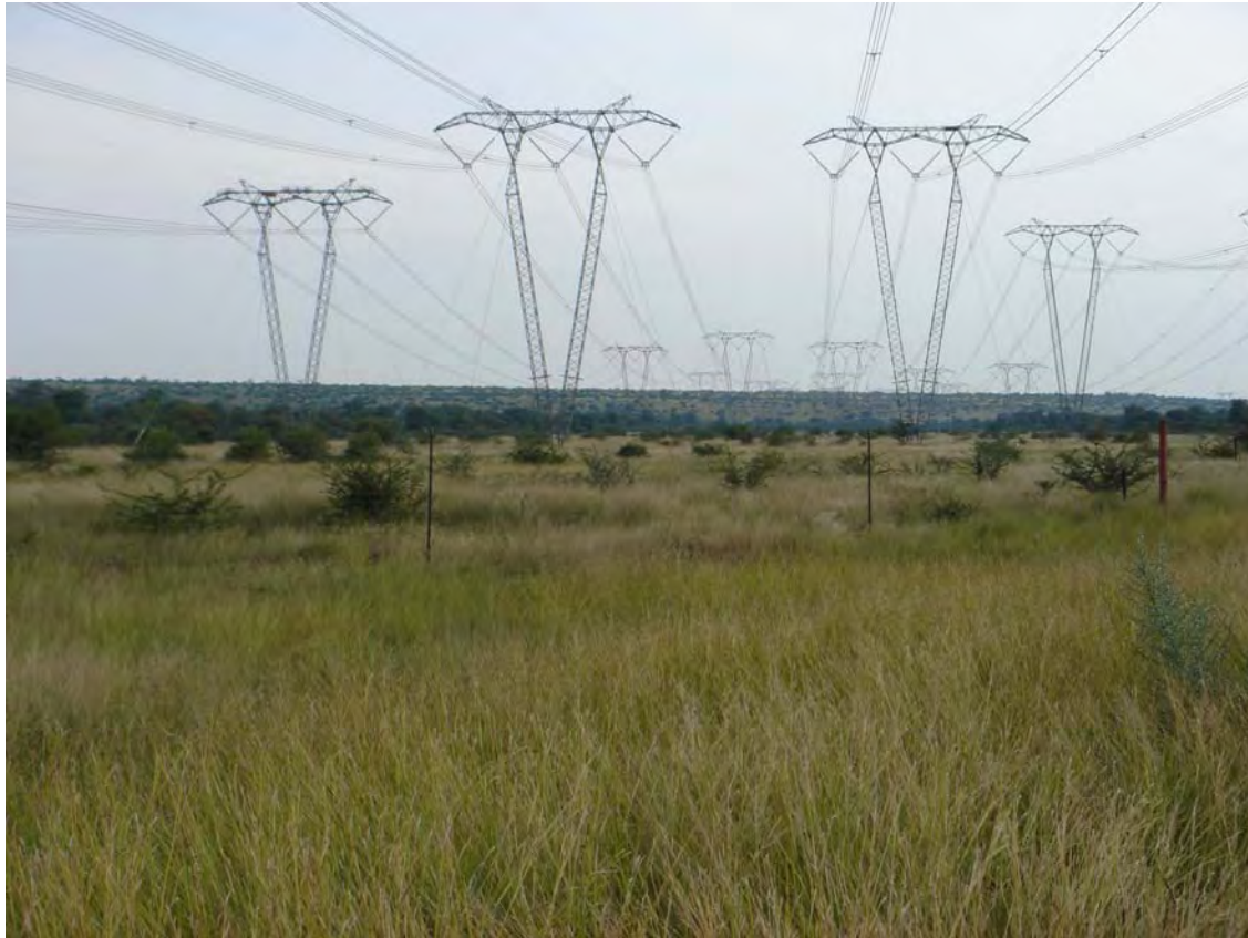
FIGURE 3.14 – 400KV TRANSMISSION POWER LINE – GUYED – V STRUCTURES NEAR MATIMBA POWER STATION
