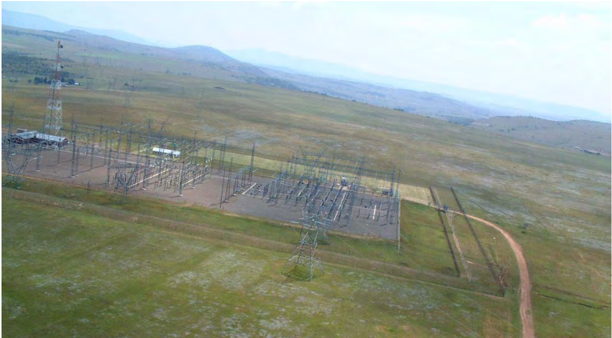
Figure 3.3 Pegasus Substation (400kV), Dundee, Kwa-Zulu Natal (note communication mast)
