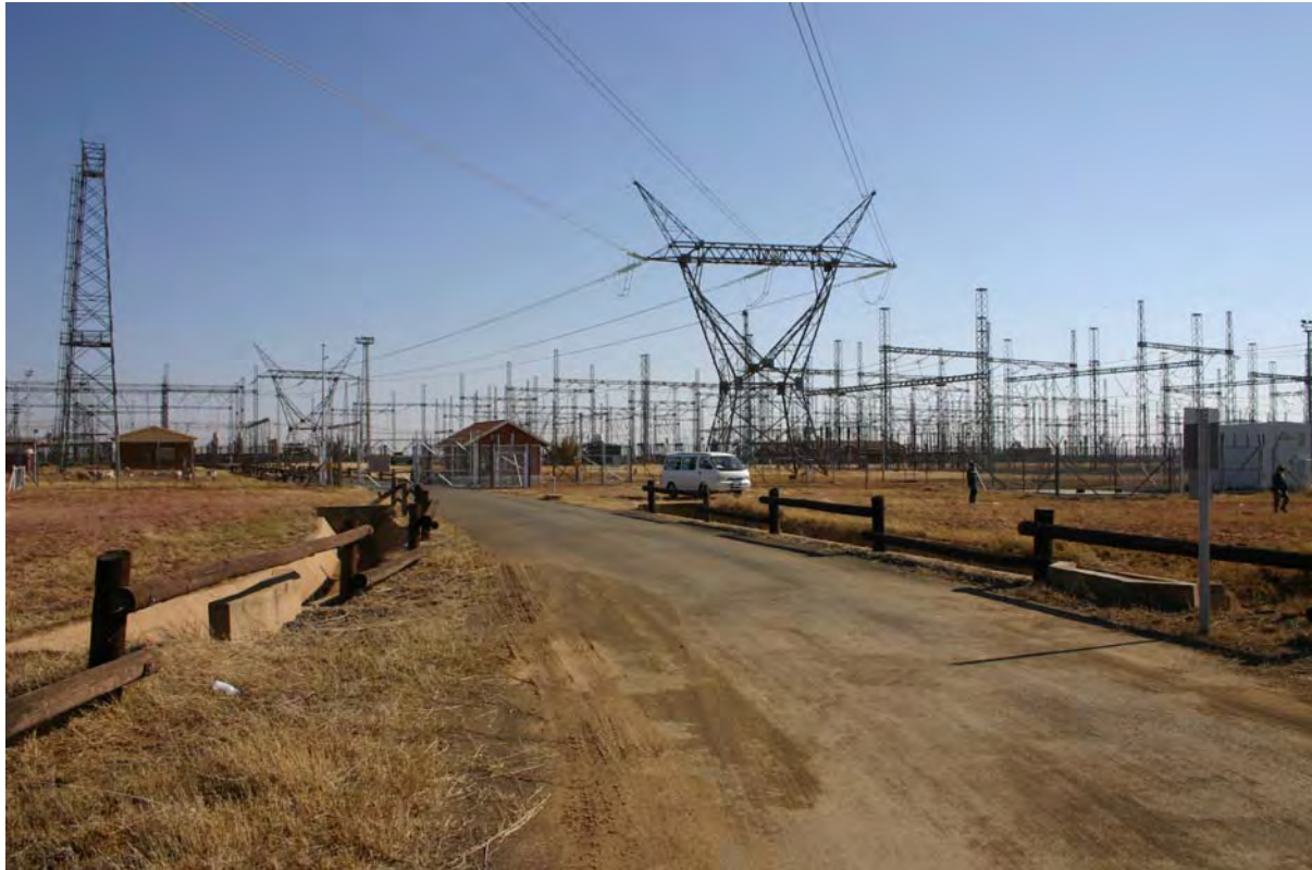
Figure 3.5. Perseus Substation (400kV), Dealesville, Free State
