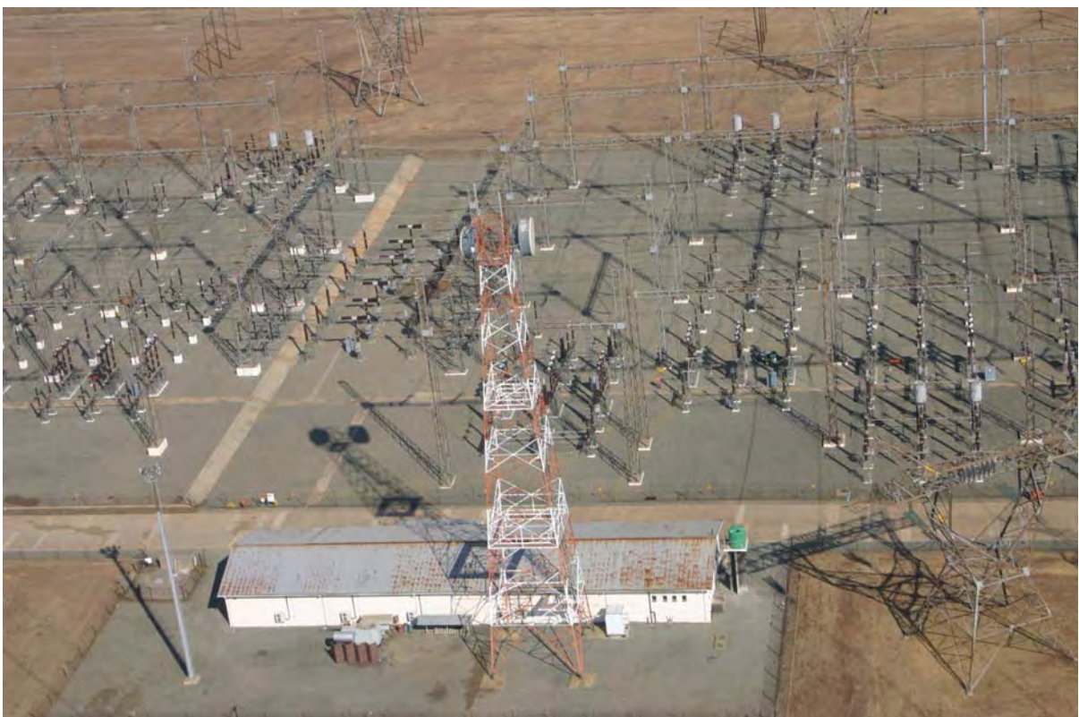
Figure 3.4. Zeus Substation (400kV), Standerton, Mpumalanga (showing communication mast)
