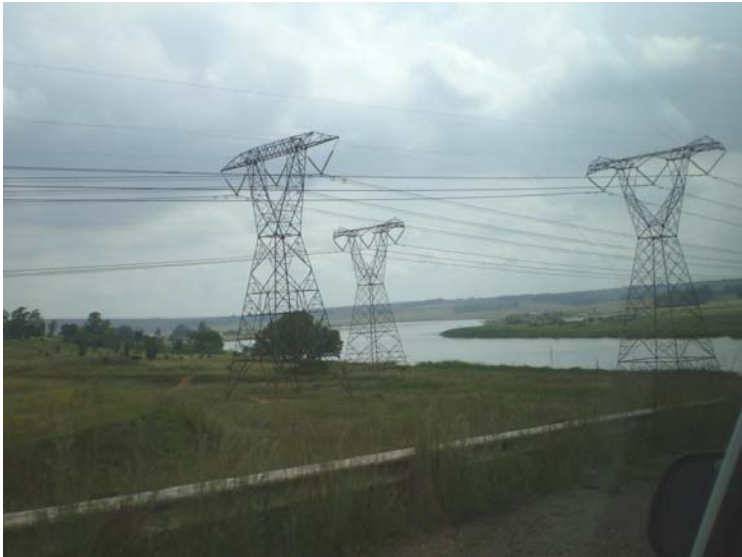
Present Self Supporting Suspension Pylons
