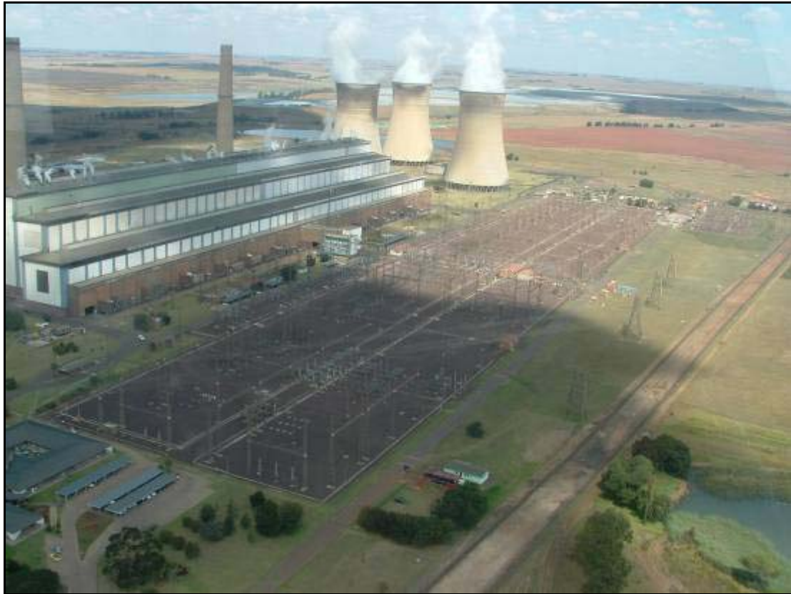
Plate 2: Aerial view of the existing Hendrina Substation
