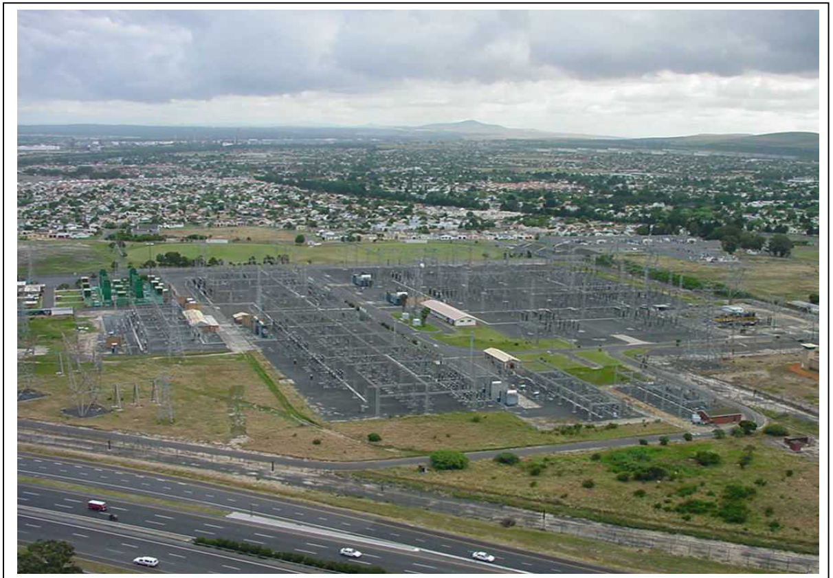
Figure 1: An aerial view of Acacia substation
