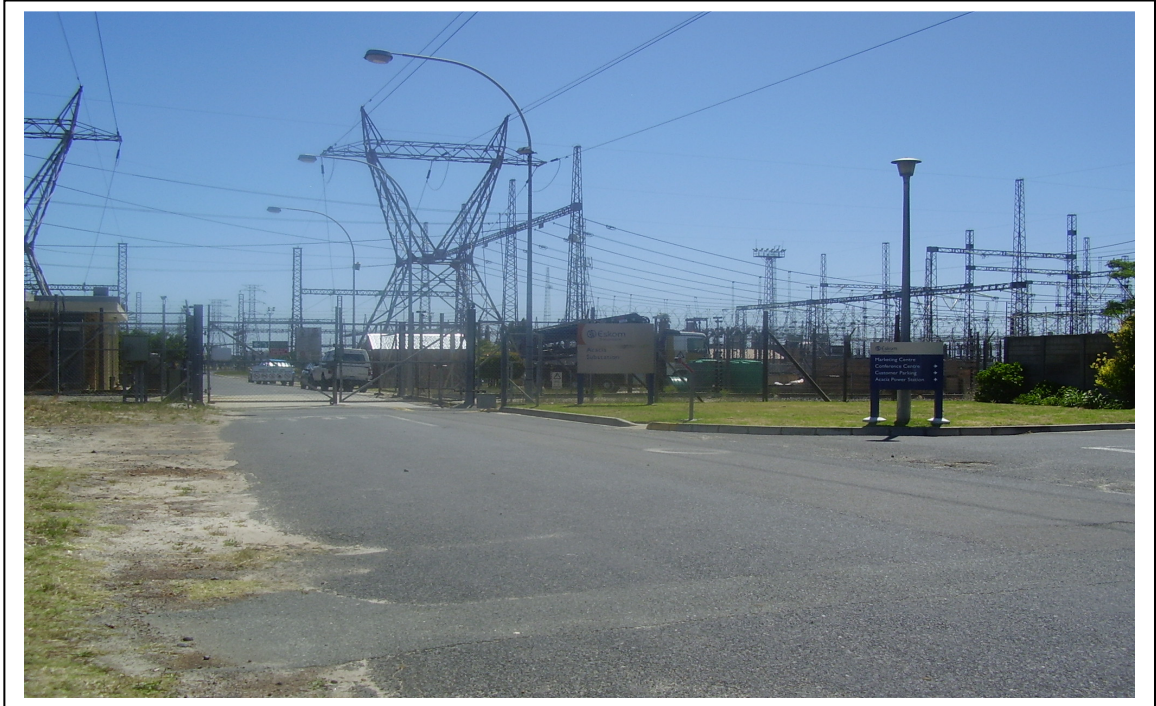
Figure 4: Picture showing the existing Acacia substation
