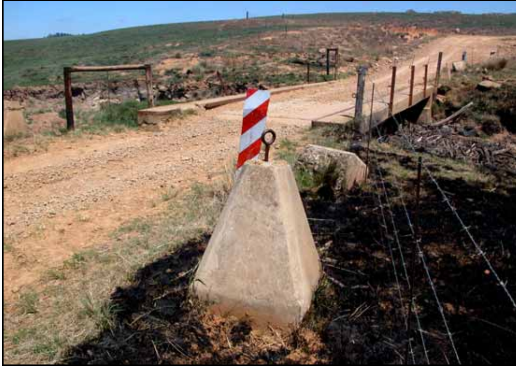
Plate 18 One of the bollards that is found at both ends of the bridge.
