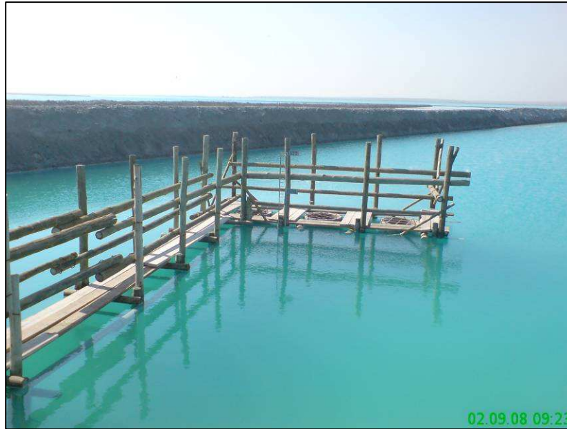
Figure 6-3: Typical Penstock Decant
