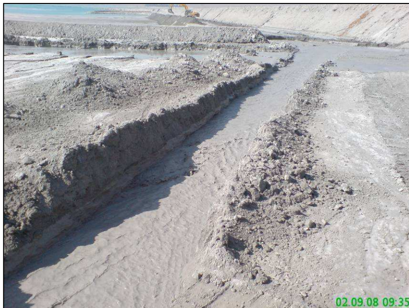
Figure 6-2: Typical Ash Distribution Channel
