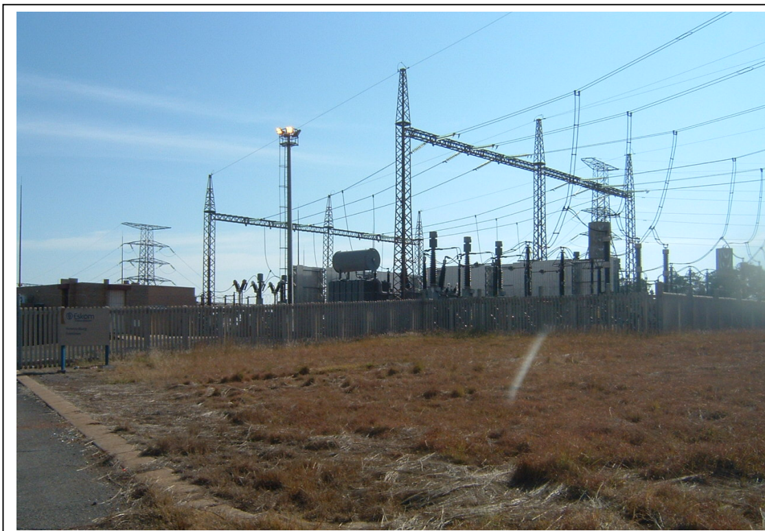
Figure 1- The Verwoerdburg and Apollo Substations are located in the southern part of the Eskom Project Area and will be upgraded (above).
