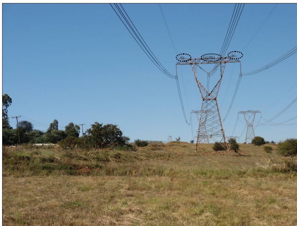
Figure 12: Bird guards (‘spikes’) fitted to a self-supporting tower.
