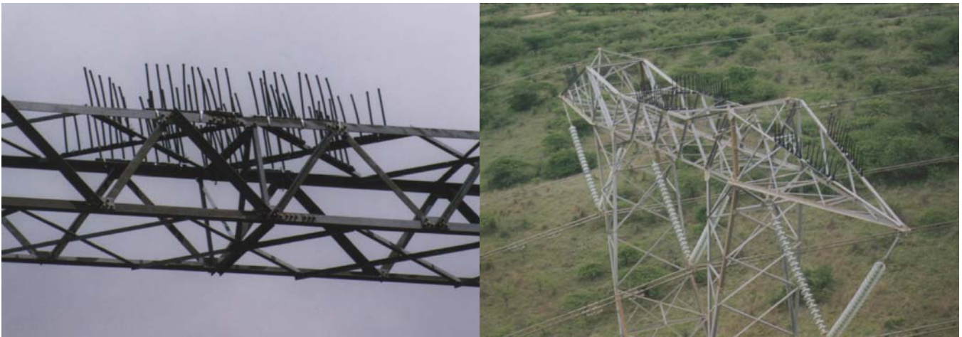
Figure 17: Photos showing the fitting of “Bird Guards” to the self-supporting tower structures.
