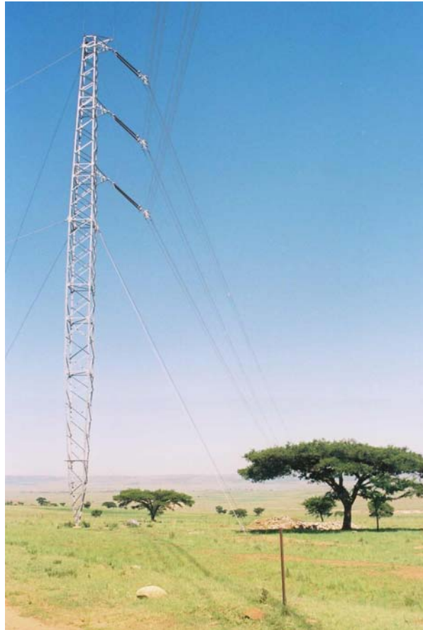
Figure 3: Example of a single pole steel lattice pylon
