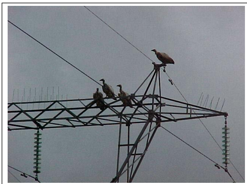
Figure 4.1: Bird guards should be implemented in areas where the streamer effect could pose a threat to the reliable operation of the Transmission line
