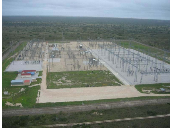
Photograph 1: Existing Grassridge Substation
