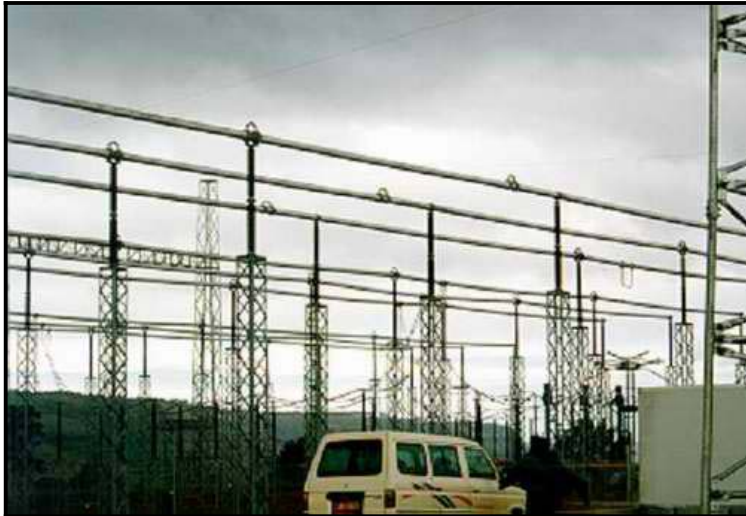
Photograph 6: Example of Tubular Aluminium Conductor Arrangement
