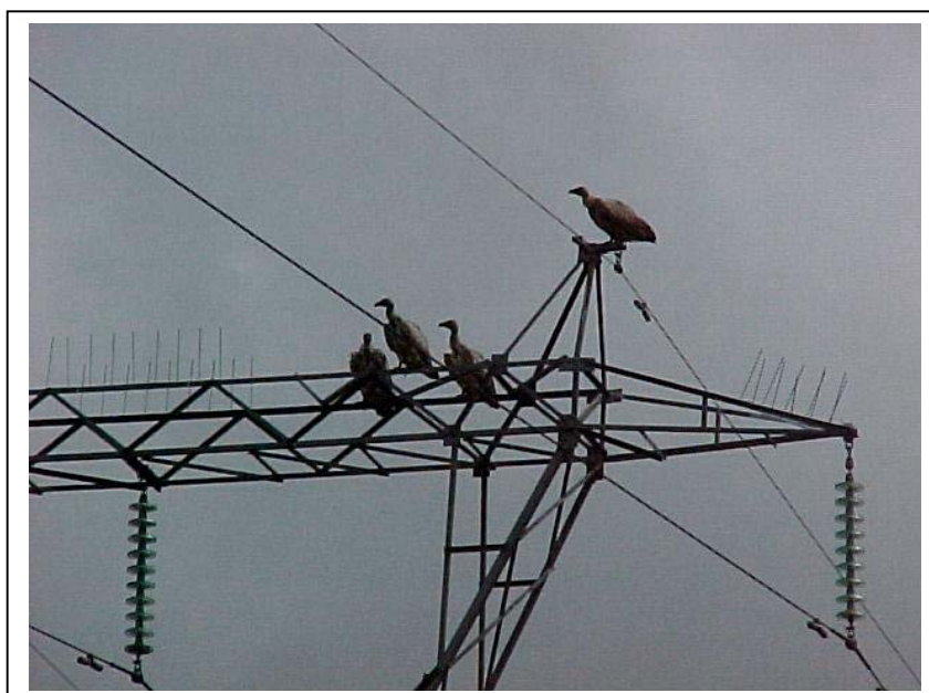
Figure 4.3: Bird guards should be implemented in areas where the streamer effect could pose a threat to the reliable operation of the powerline
